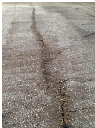
Cracks in the facing visible after hydrodemolition
